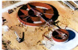
DAVCO™ Field Erected Treatment Plants
