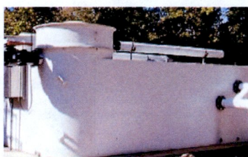
Deep-Bed Sand Filters
