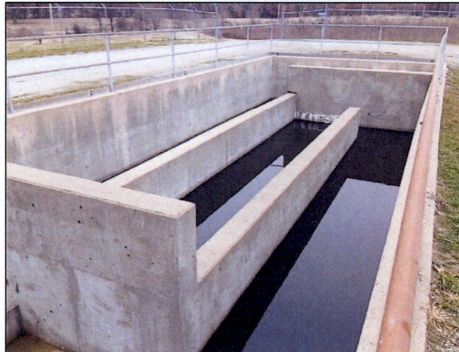
Figure 14.0: Photo of Existing Disinfection Basin
