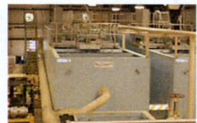
NxClear® Denitrification Filters
